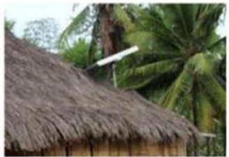
Solar Home System
